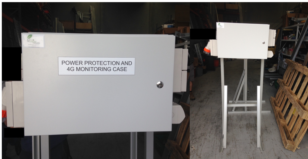
Power Protection and 4G Monitoring Case Mounted on a Frame
